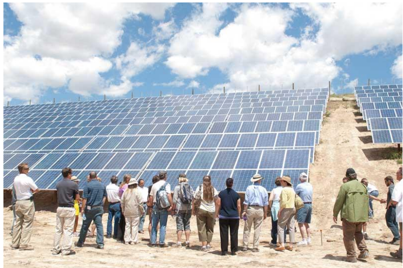
Garfield County Airport Community Solar Array, near Rifle, Colorado
